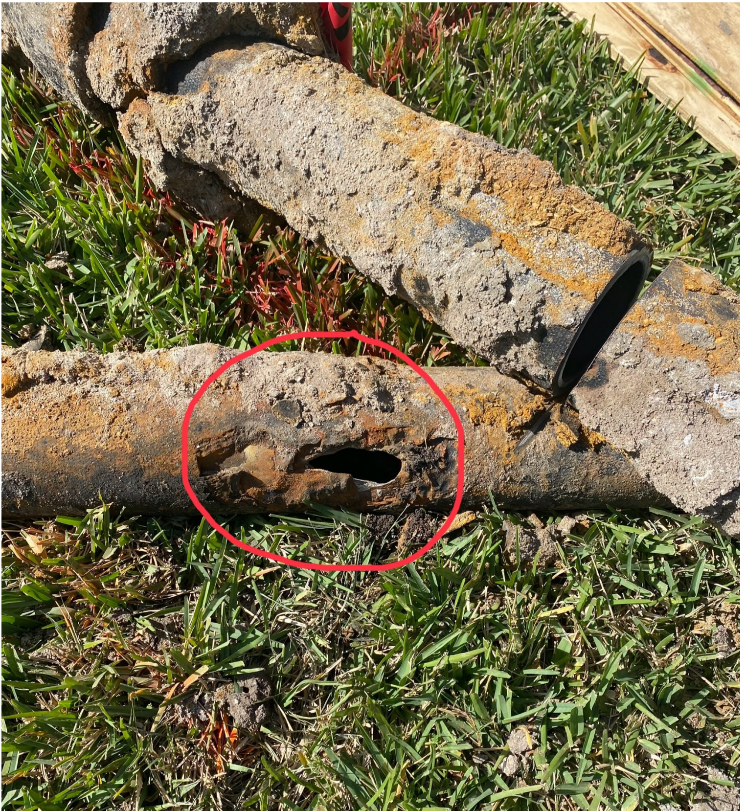
Building 108 Pipe Break
